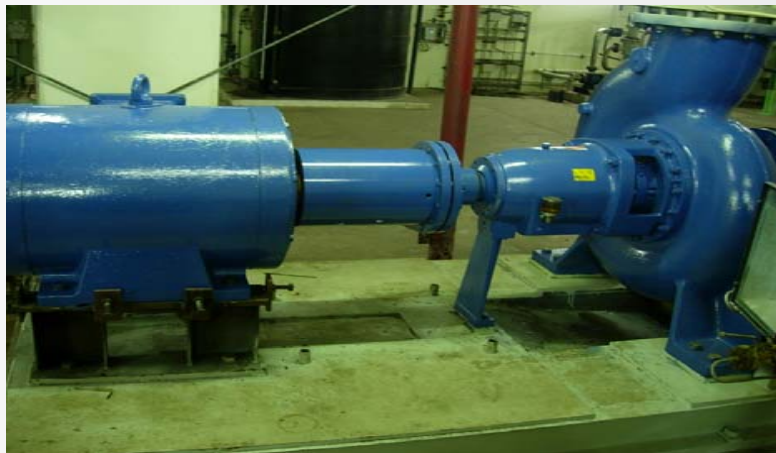
Secondary Cooling Pumps
