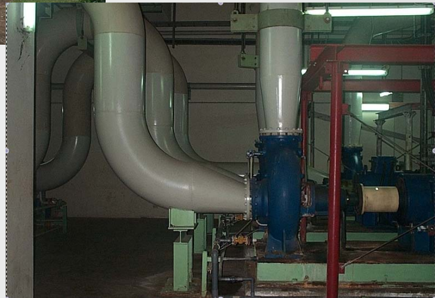
Secondary Piping System
